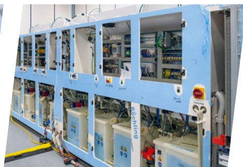
The system's electronics are housed at the upper end of the back, whilst the lower section contains the storage tanks for liquids such as acids, bases and solvents.
